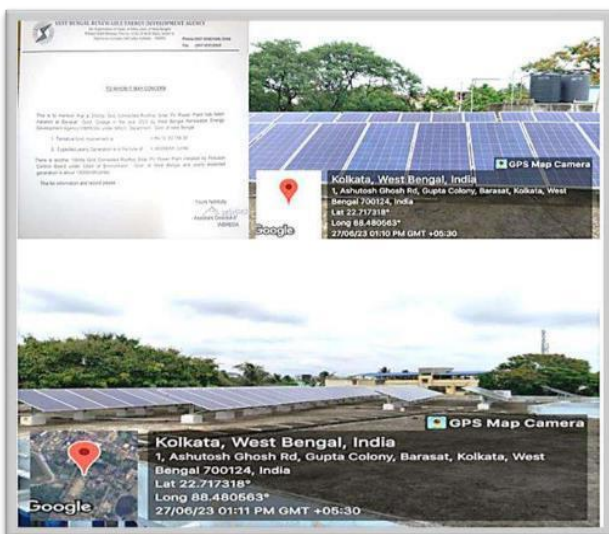
10kWp and 20kWp rooftop Solarpower units
